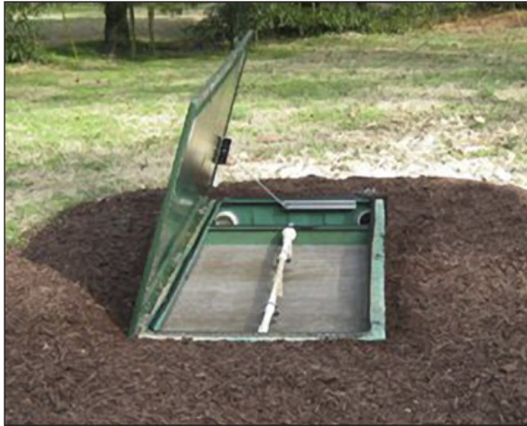
This AX20-RTUV with Ultraviolet Disinfection, engineered by Kevin Davidson, is the first to be approved by the North Carolina Department of Water Quality for a surface discharge permit.
