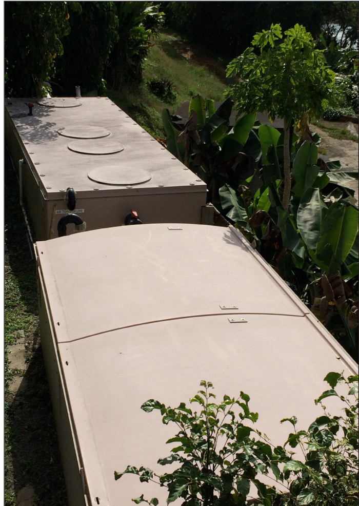
The Mountain Top condos use a T-Max tank for primary treatment, followed by a 4.3-meter (14-ft) AdvanTex AX-Max Treatment System. Together, they handle up to 11.4 m 3 /day (3,000 gpd).
