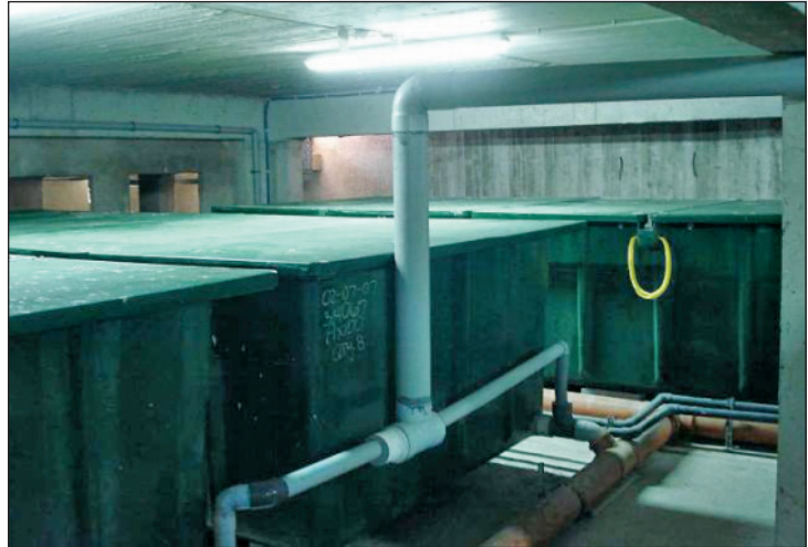
St. Constantin's engineering firm – Dialynas S.A. – designed an innovative and compact interior wastewater system.
