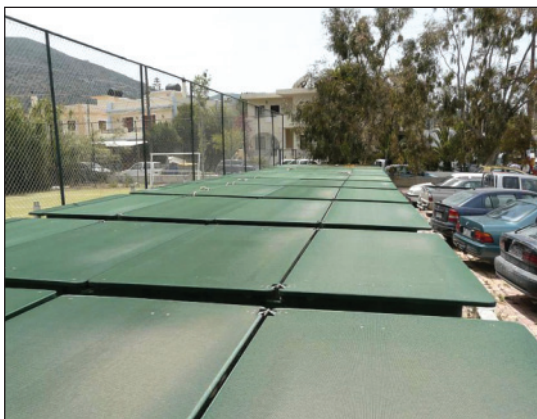
After initial installation, the treatment system was relocated to an area next to the parking lot in order to accommodate hotel expansion.
